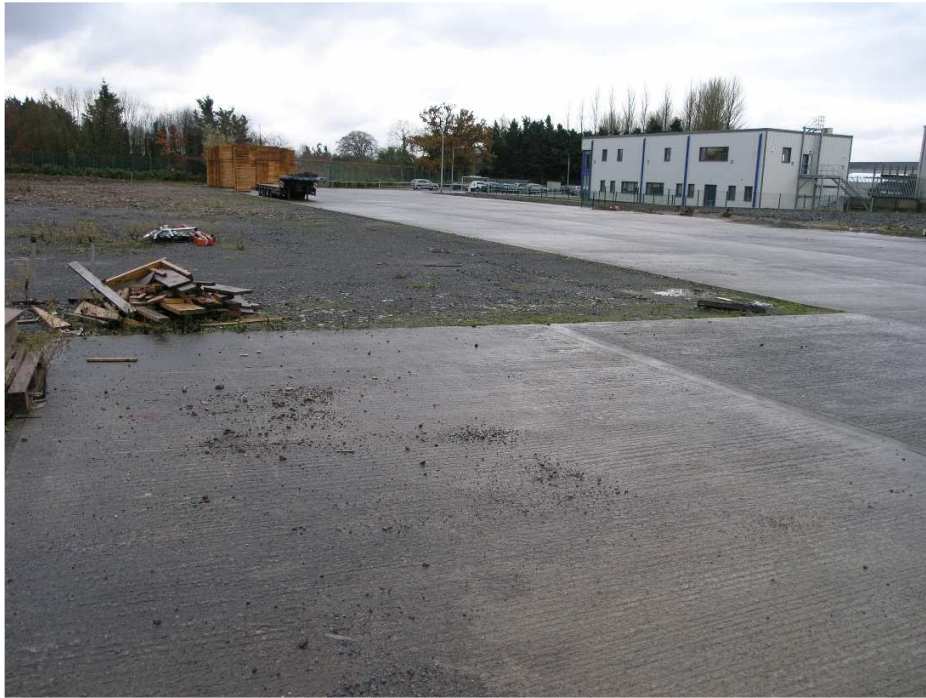
Figure 11.10: Existing concrete surface along west and north side of the development area (looking east)
